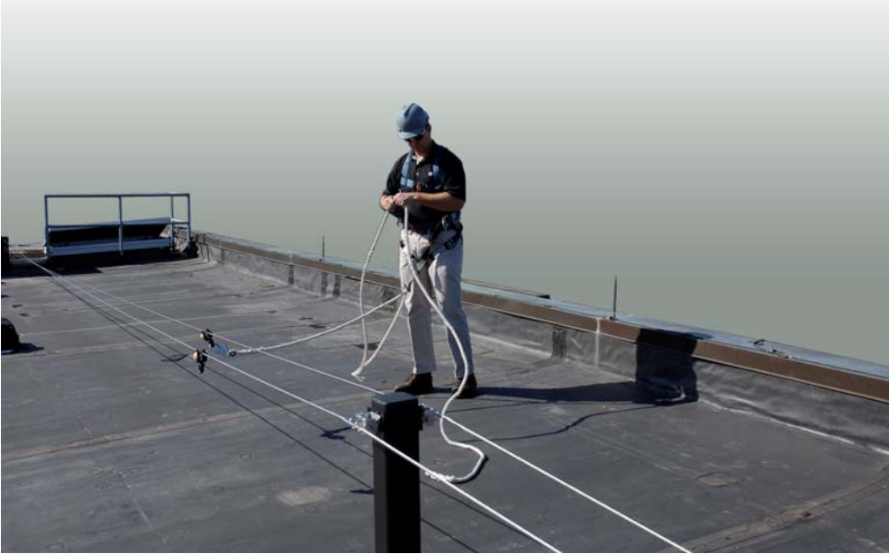
Exhibit 3 - This HLL system protects workers near the roof edge.
