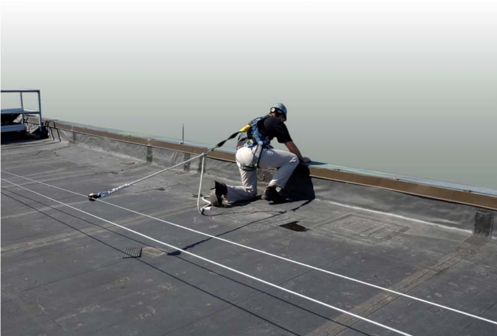
Exhibit 4 - This HLL system protects workers performing tasks at the roof edge.
