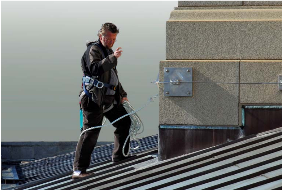
Exhibit 5 – This photograph illustrates how HLL systems can be effective at providing continuous fall protection around corners.
