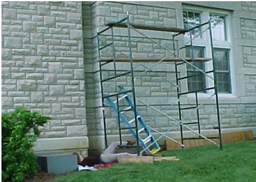
Exhibit 4. Scaffold violations contribute to worker fatality.
