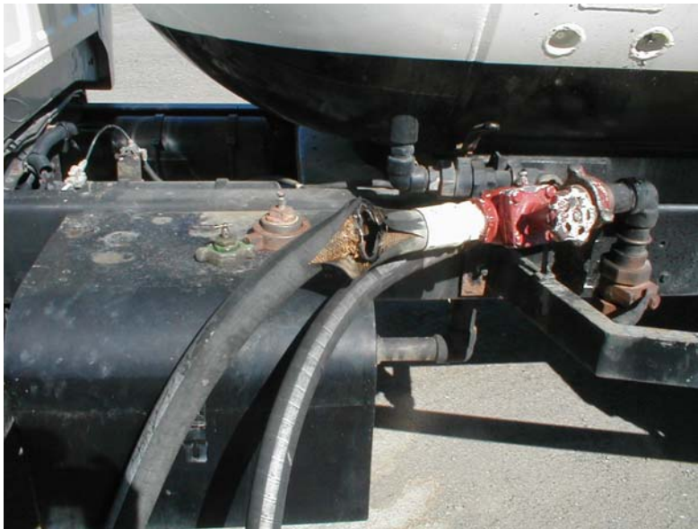
Ruptured Ammonia Hose Maximum Working Pressure: 350 psi v Stainless steel reinforced
