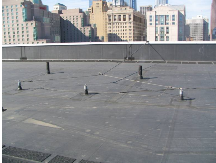
Exhibit 5. This photo shows permanent roof anchorage points. By designing fixed, structurally sound anchorage point workers will have convenient tie-offs during construction and future maintenance.
