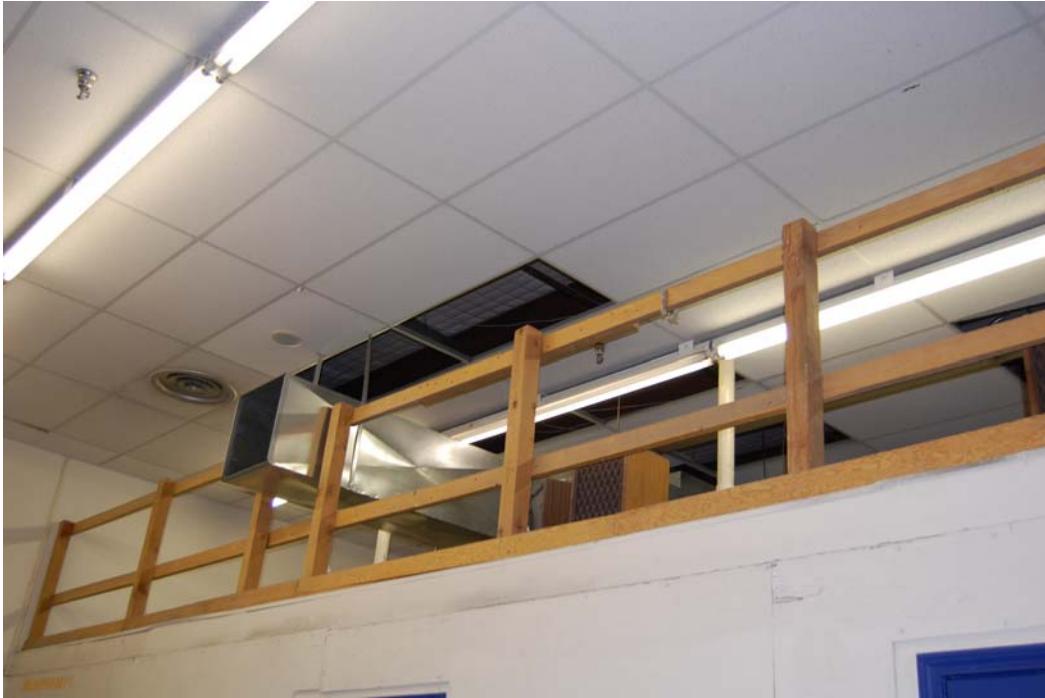
Exhibit 3. This photo shows guardrails along a mezzanine. Guardrails prevent fall injuries when working near open side floors or platforms.
