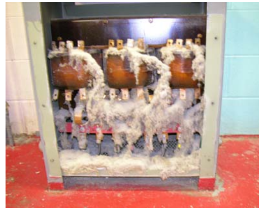
Figure 13. Dry Transformer Blocked with Dryer Lint
