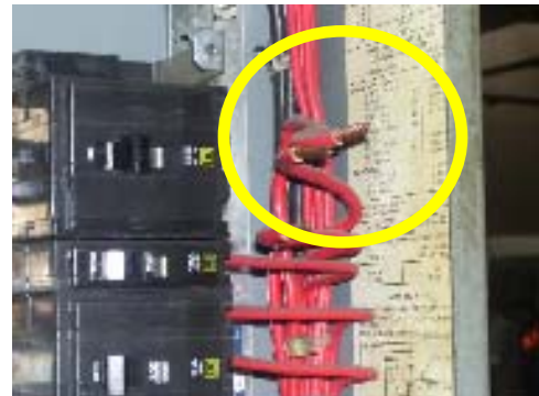
Figure 6. Exposed Wires OSHA 1926.403(e)
