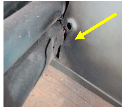
Figure 18. MCC Feeder Rubbed and Shorted
