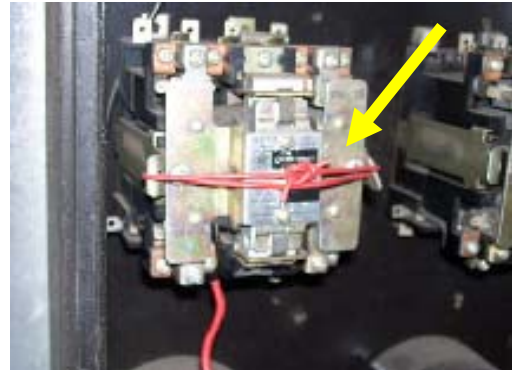
Figure 5. Component held in place with wire knot. (NEC 110-12) Not Installed in Workman-like Manner
