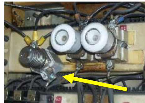
Figure 23. Broken Fuse (NEC / OSHA)
