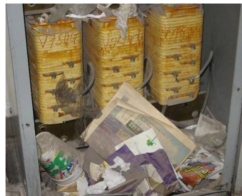
Figure 12. Combustible Dirt and Debris
