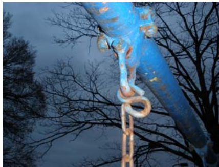
Figure 14. Regular inspections must be conducted to discover hazards such as this faulty "S" hook.
