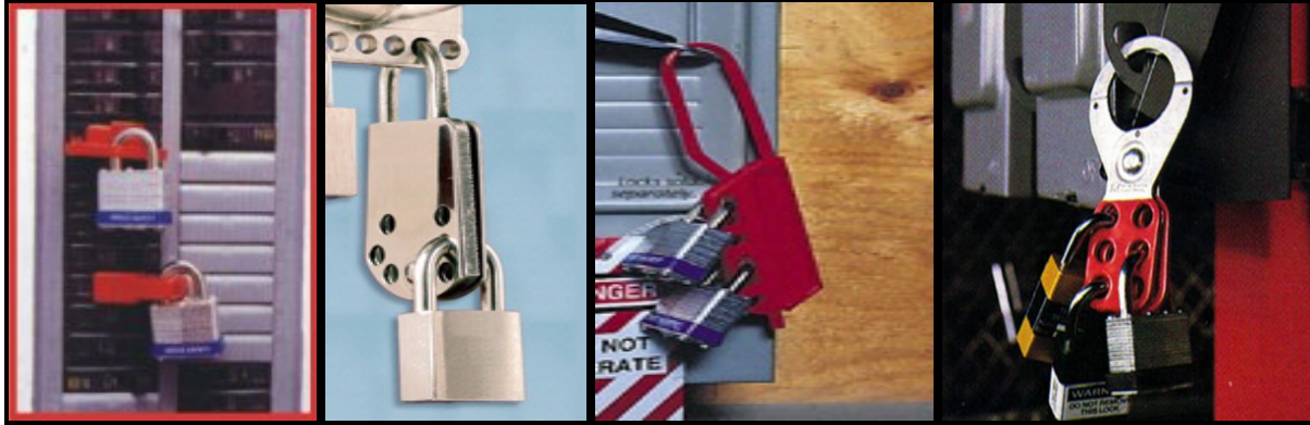
Figure 6. Electrical Panels Shown “Locked Out”
