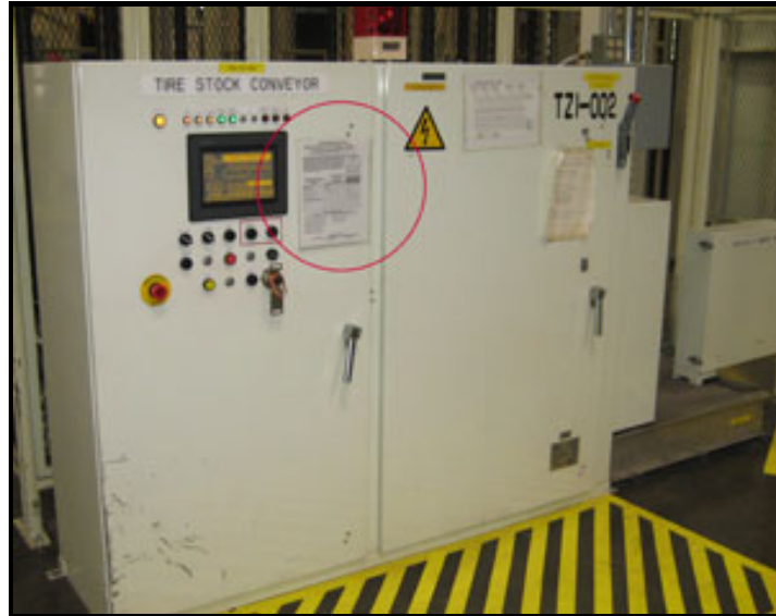
Figure 10. Equipment-Specific Energy Isolation Procedure shown in file on front of Equipment Control Panel.
