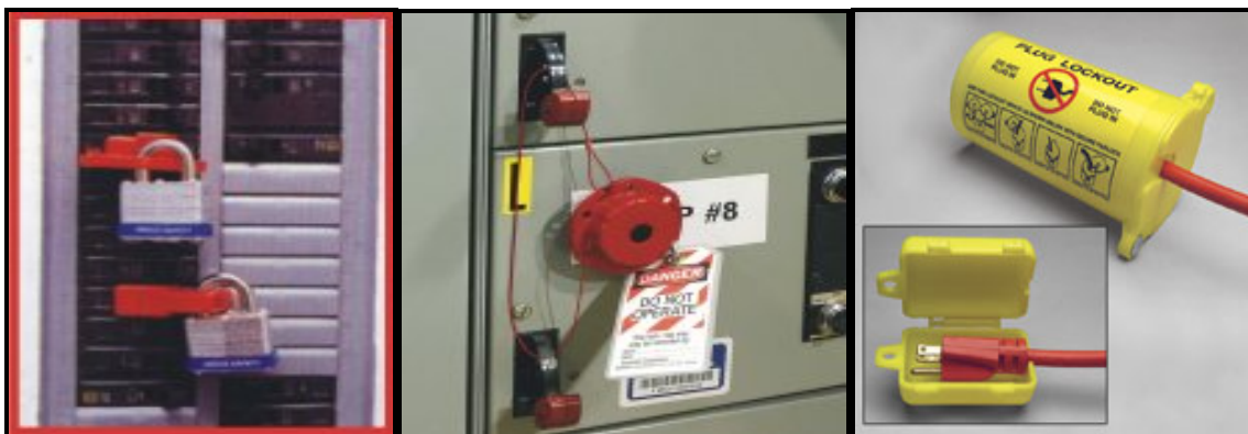
Figure 1. Locks and Tags on Single and Multiple Electrical Breakers: Electrical Plug Lock Box
