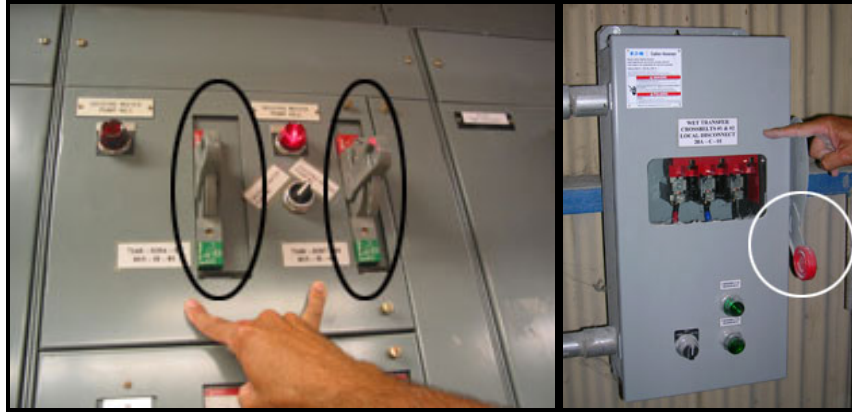
Figure 4. Disconnect Panels with “Lockout Here” Label and Energy Isolation Information
