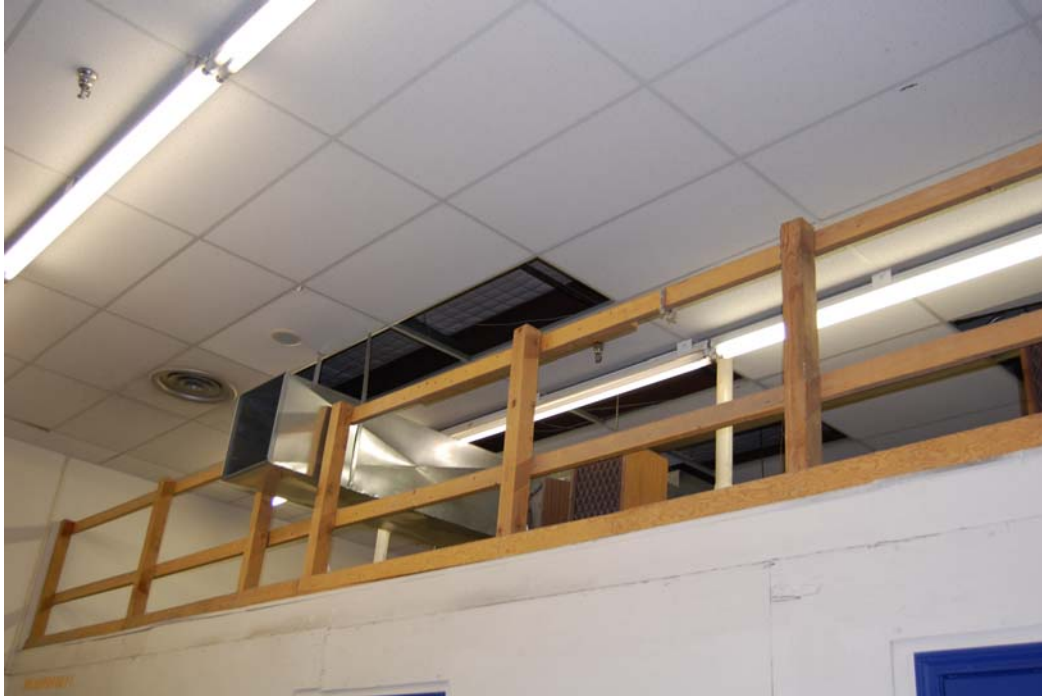
Figure 1. This photo shows a guardrail along the open side of a loft used for storage.
