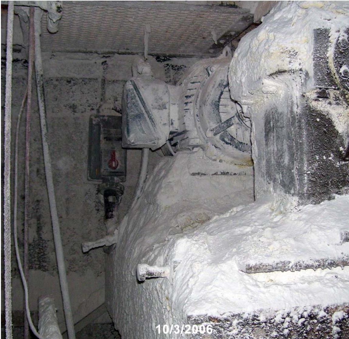
Exhibit 4. Housekeeping conditions such as this may lead to a major loss incident. (Photo courtesy U.S. Chemical Safety and Hazard Investigation Board.)
