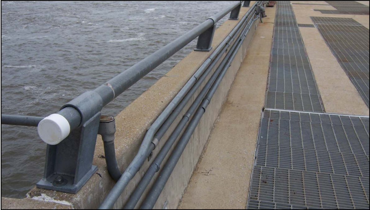
Exhibit 2. A primary focus for USACE is for initial design to account for fall protection measures. This wall required retrofitting with a handrail since it was not tall enough to be compliant.
