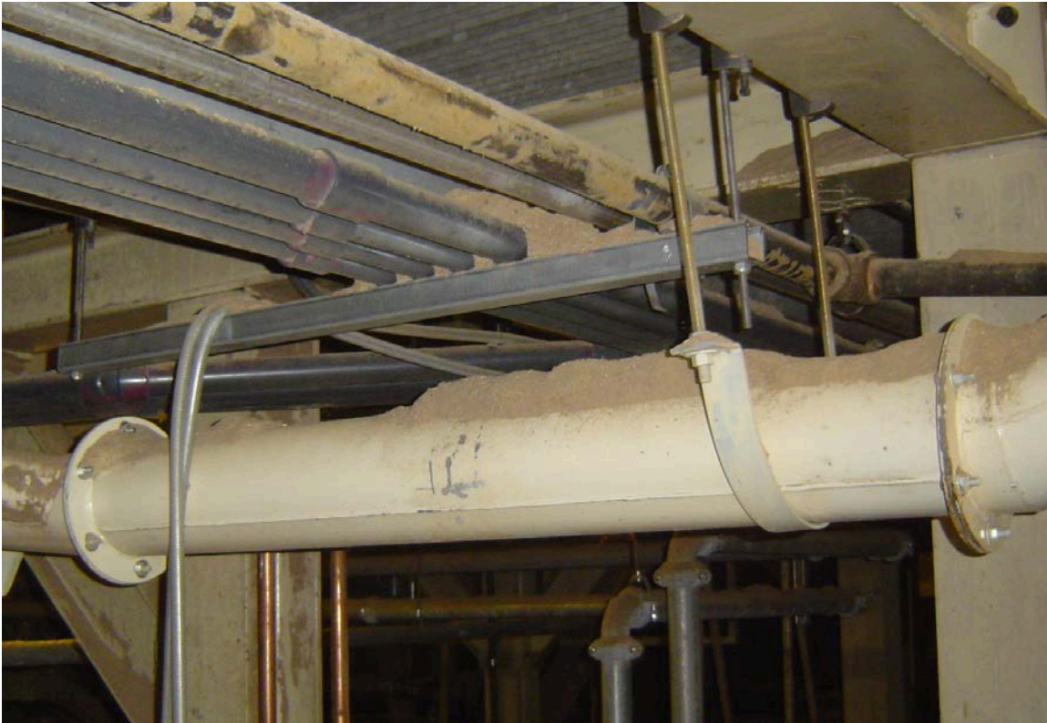
Exhibit 3. Ducts, conduits, and building members should be maintained free of dust accumulations.
