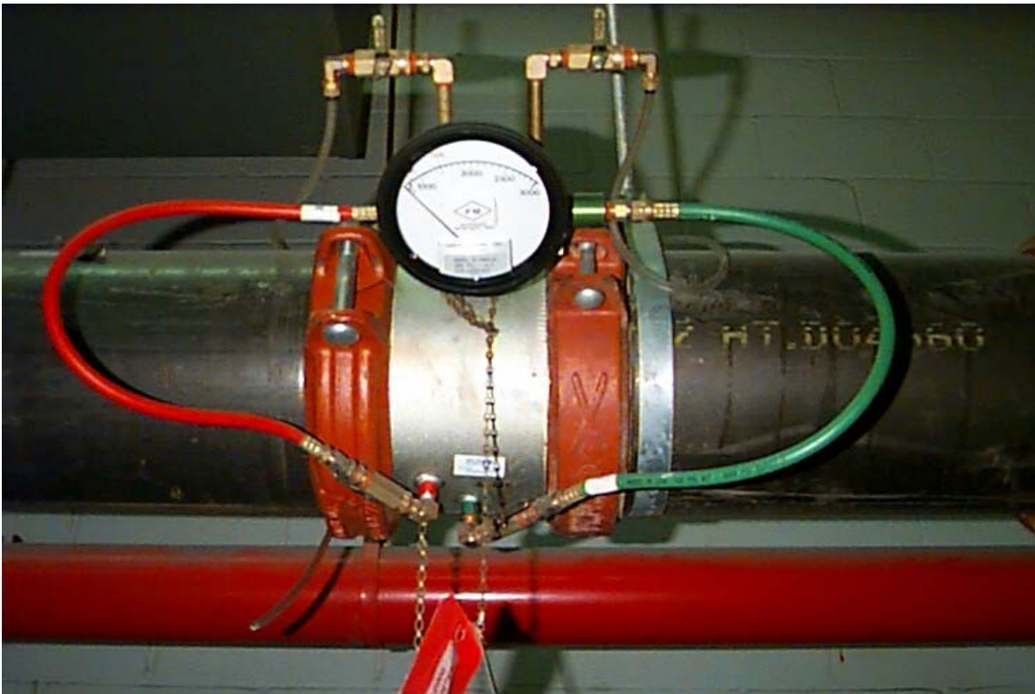
Exhibit 9. Testing Flowmeter by Use of Bypass Flowmeter
