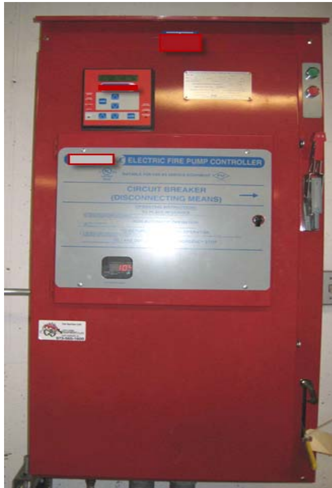
Exhibit 4. Electric Pump Controller.
