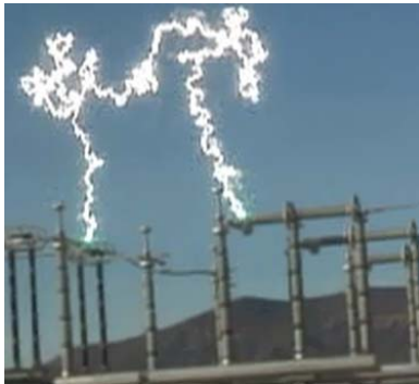
Figure 10. Example of one pole of 3-pole circuit failing to open
