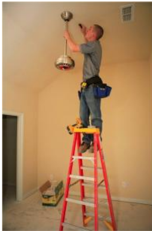
Exhibit 2. Making ladder work though not the proper length
