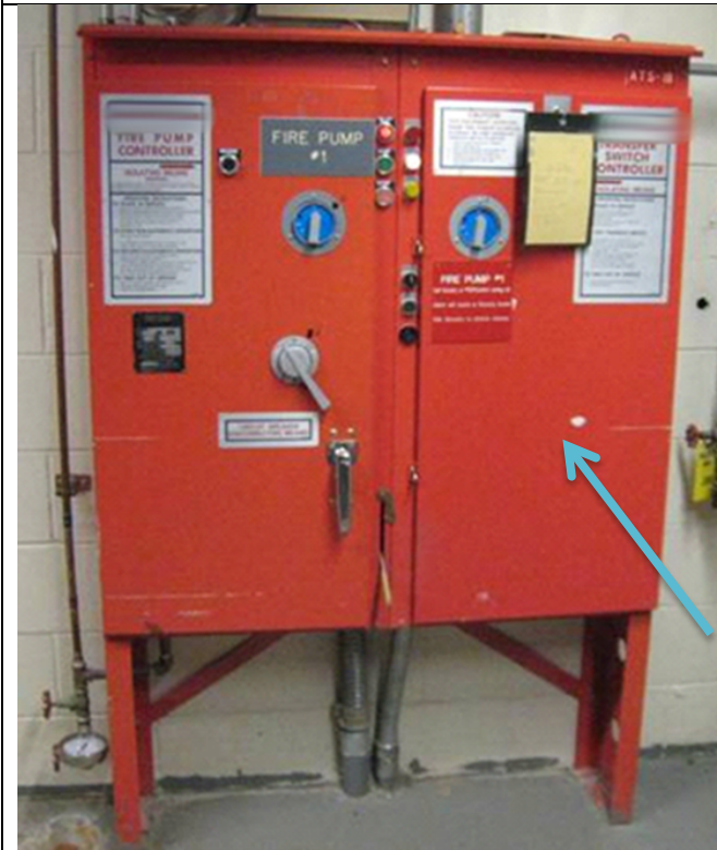
Electric Fire Pump Controller with Automatic Transfer Switch (blue arrow). If the fire pump is connected to a secondary electric supply via a transfer switch at the fire pump it should be tested as per NFPA 25. Monthly under a “no-load” condition and annually during the pump test. During the annual pump test the transfer switch is operated while the pump is operating at 150% of its rating. Power must switch automatically and the pump continues to run on emergency power. Pumps readings must be taken when the pump is operating on emergency power. The readings are compared to when the pump is operating on utility power.
