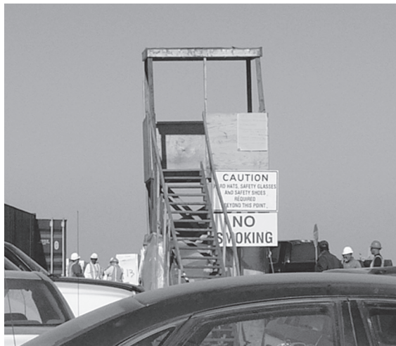
Photo 3 (left): The tower was used to count the refrigerators when they could not be seen well from the ground. The site safety manager also used the tower each day to survey the site before beginning a walk-through inspection.
