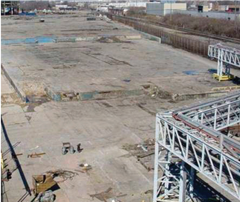
For the automotive components manufacturer, the design called for leveling all 29 structures.
