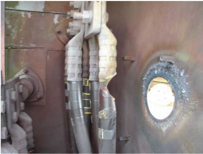
Photo 2: The arc in this case lasted long enough for sufficient heat to develop to melt the steel enclosure.
