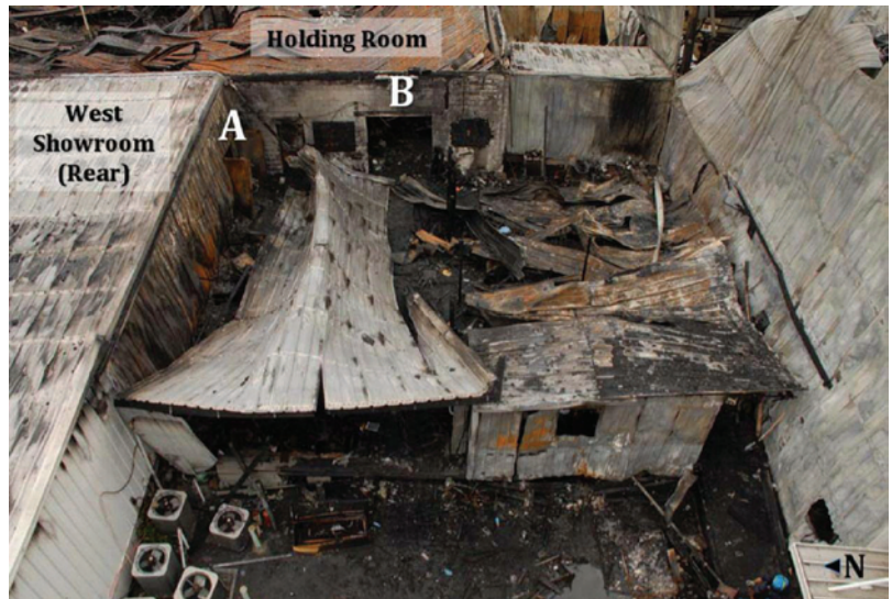
Photo 7: Photo shows total collapse of the loading dock area. Fire penetrated through unprotected wall openings and through wall construction materials to spread in three directions.
