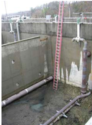
Photo 1 depicts a permit-required confined space that is not enclosed. Failing to recognize such a space places workers at risk.
