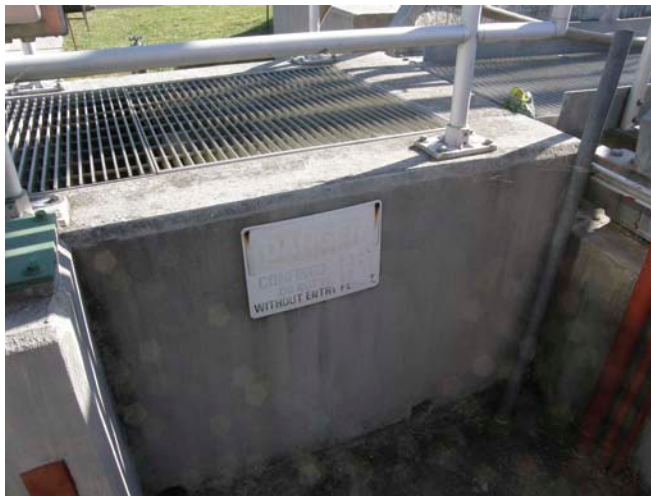
While signs are a good way to identify PRCS, they should not be the only method used since signs fade (Photos 2 and 3) or get damaged, and spaces get overlooked.
