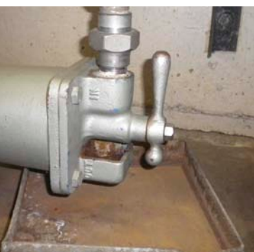
Photos 3 and 4: Typical condensation drip traps.
