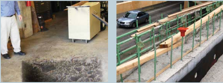
Photo 3 (left): Identified fall exposure to employees from permanent hole. Photo 4 (right): Exposure to unprotected rebar, presenting an impalement hazard.
